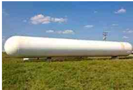
High Pressure Tank
